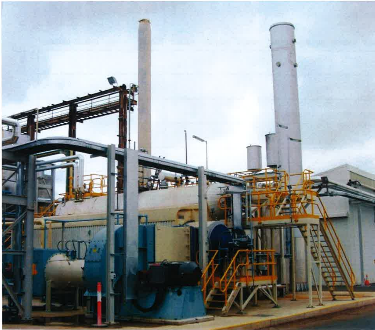
New boiler at Australind. To be commissioned in late 2013.
